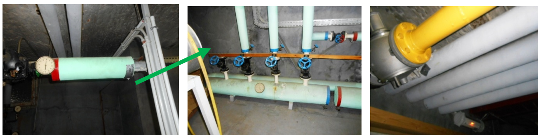
photo: 1, calorifuge (plâtre (isolation))
