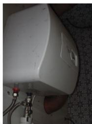
boiler escalier cave>evier cuisine
